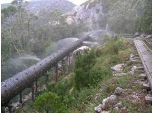
Leaking King Billy woodstave pipeline in 2007
