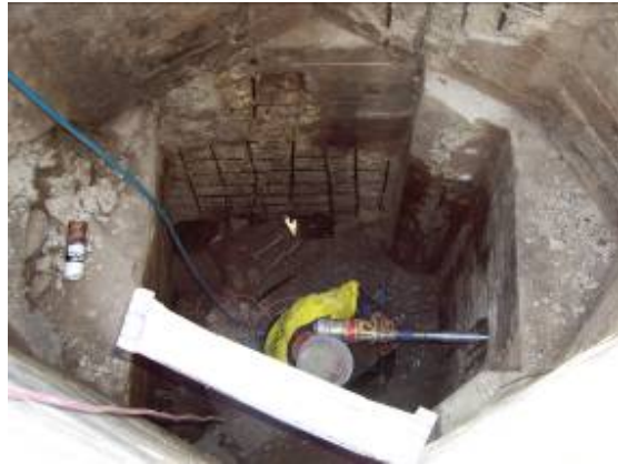
Figure 5: View inside chimney with flue bricks removed, showing typical extent of reinforcement corrosion.
