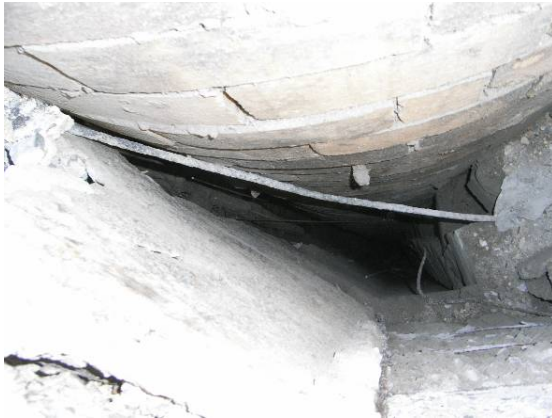
Figure 4: View down the chimney from the top with c.1980's cap removed showing the general extent of delaminated, friable concrete.
