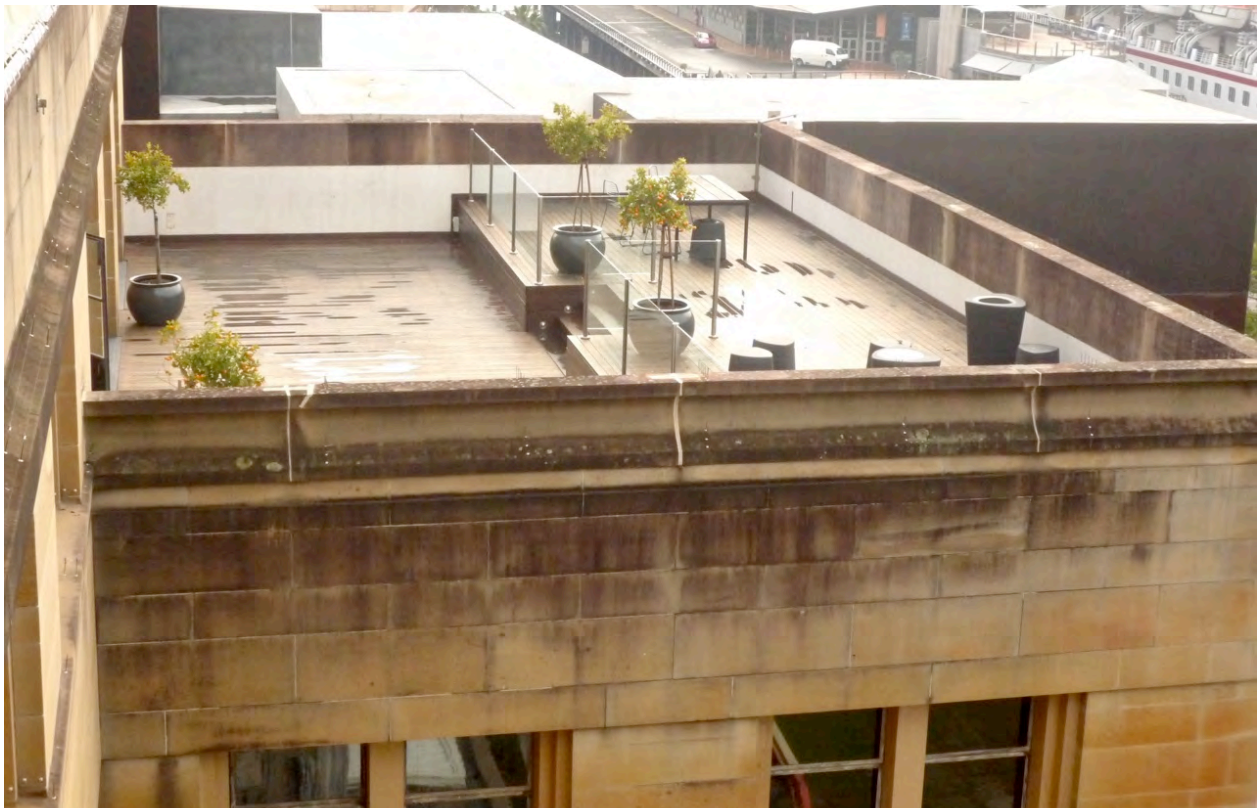
Figure 1 View looking north over the northern balcony of the Museum of Contemporary Art building. Trials were conducted on the inside faces of the very large parapet stones to the north, east and south walls of the balcony.
