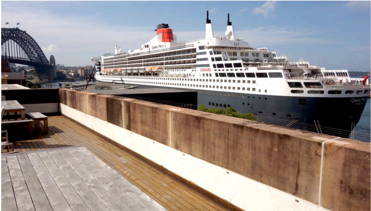
Figure 2 The eastern wall of the balcony, 23 months after treatment. The dark area left of centre is the untreated control panel; to its left are panels treated by poultice application of biocide. Note the wide zones around the mortar joints showing a biocidal effect, and the evidence of previous cleaning in the form of horizontal bands from pressure-washing.
