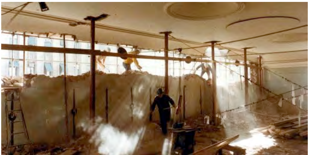
Fig.3 – Demolition in progress on the upper west wall of the former Legislative Council Chamber c1978, showing the extent of intervention carried out at the time ( History SA )
