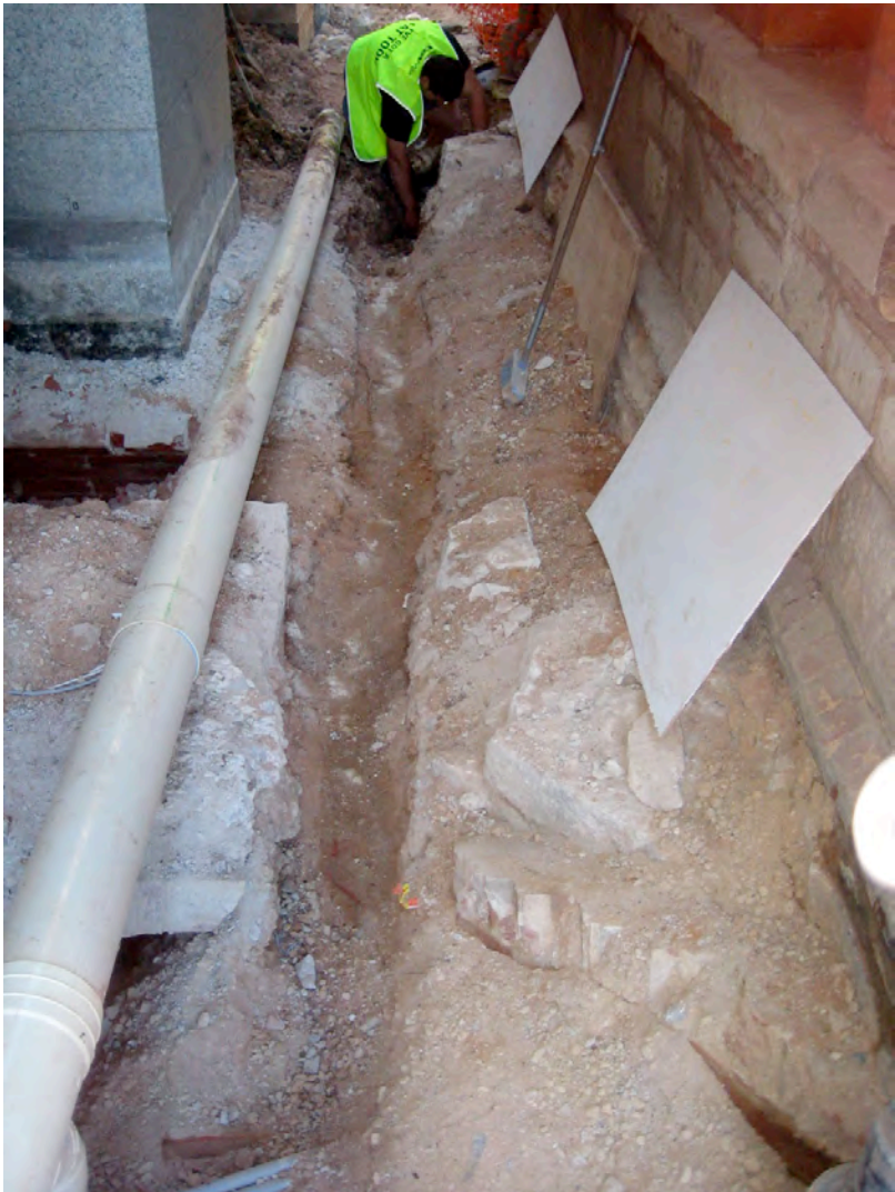
Fig.4 – Service excavations revealed the footings of the former east bay window which required diversion of the services (Swanbury Penglase 2012)
