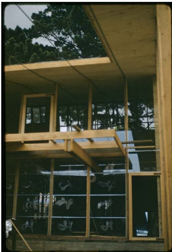
Figure 5. Courtyard elevation of the Boyd House while under construction in 1958. Note the fresh yellow Oregon timbers. (Peter Wille, Collection of architectural slides, State Library of Victoria)
