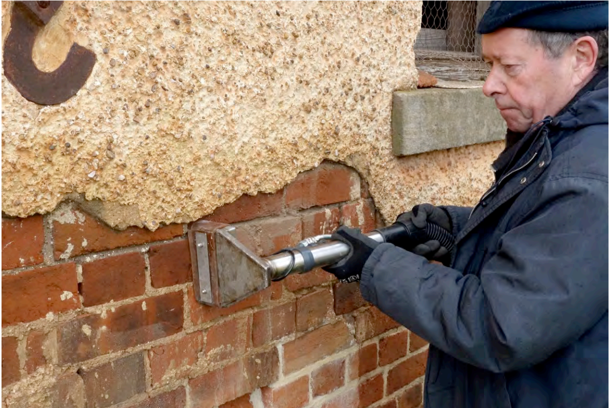
Figure 1 Captive-head washing system being used by Walter Heim to remove dust and dirt from brickwork prior to render repairs at Brickendon, Longford.
