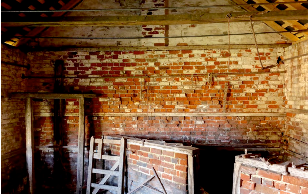
Figure 3 Interior of northwest wall showing extensive decay of low-fired bricks due to salt attack. 8.8 m 2 of the wall was treated with two passes of captive-head washing.
