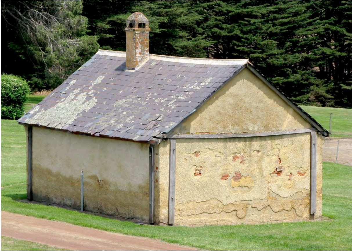
Figure 2 Woolmers Estate blacksmith's shop from the north. Failed roughcast rendering on the northwest wall (to the right) is allowing penetrating dampness to carry salts through the 350 mm brickwork to the interior (see Figure 3).
