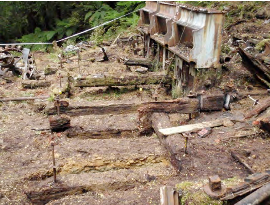
Figure 3: Lord Brassey stamper battery foundation condition 2012 (Jim Staton)
