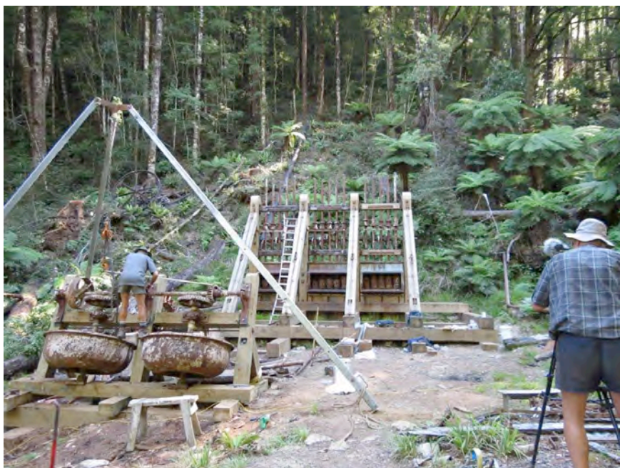
Figure 5: Lord Brassey battery, Jim Staton tightening the last nut, shear legs positioned above the berdans.
