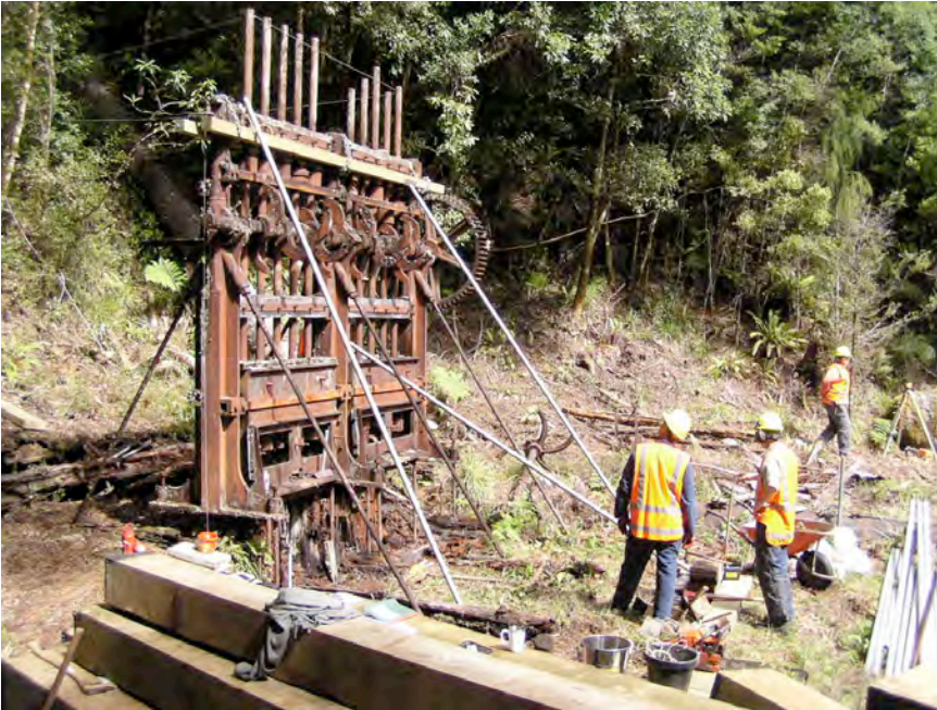
Figure 2: The Golden Lead stamper battery prior to restoring the foundation timbers in 2008 (Jim Staton)
