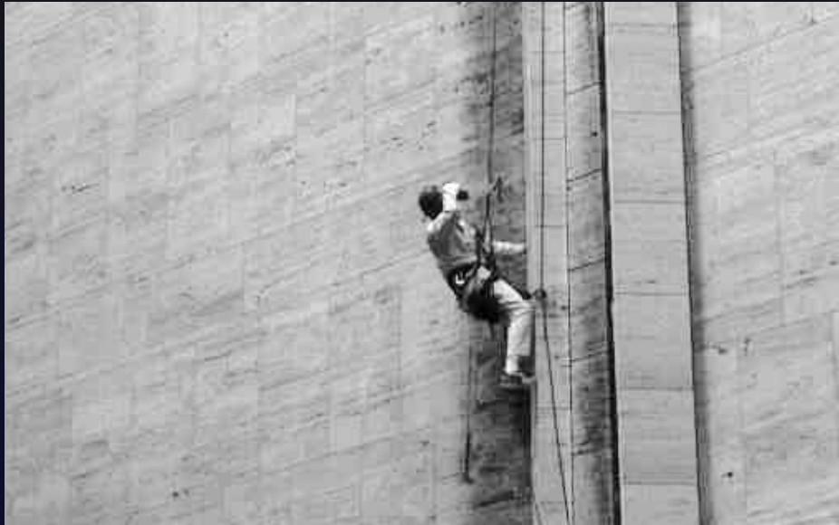
Lincoln Center for the Performing Arts - New York State Theater, Industrial Rope Access during "Close-Up" Travertine Inspection
