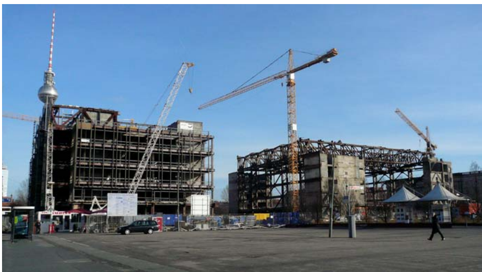
6. The demolition of the Palace took a long time from 2006 until 2008, photo: January 2008 (© Lars Kinder)
