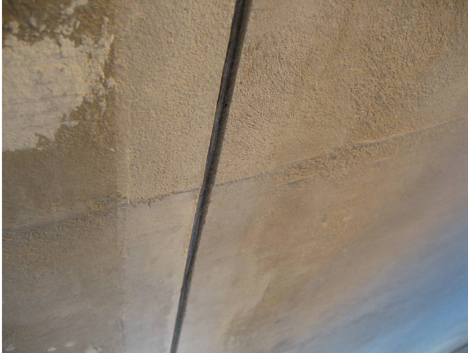
Fig. 5: Patches carefully recreated the texture and board-form marks. This patch is at the sixth floor ramp wall, where vertical control joints remedially installed during the 1992 work were retained.
