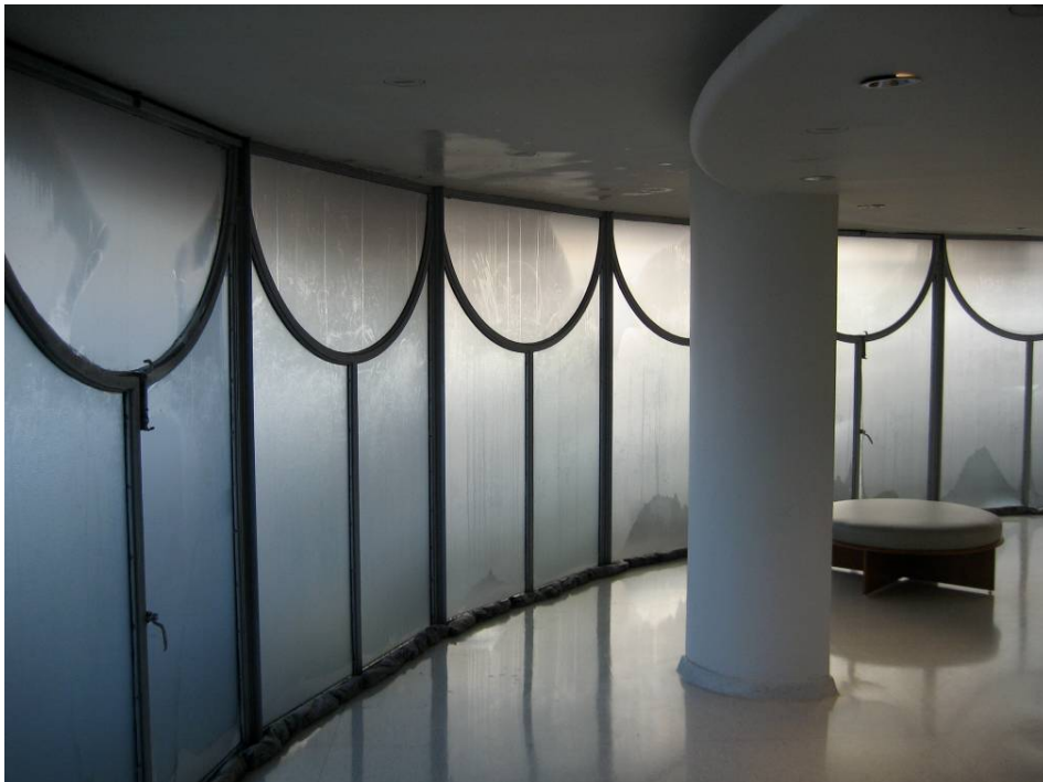
Fig. 6: Excessive condensation was an issue and the reason for not retaining the original single-glazed windows and skylights.
